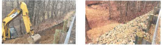
County crew repairing a road slip on Colony Rd., C.R. 74 in Fox Township
