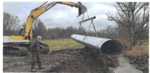
County crew replacing a culvert on Arbor Rd., C.R. 14 in Augusta Township.
